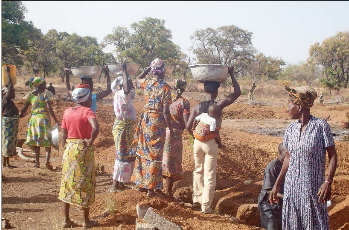
Villagers work together on the foundations for the Community Center Project at Nyobok-Nkunzesi in Northern Ghana, 2012. The health clinic, funded in part by the Rotary Club of Kelowna-Ogo-pogo, was the priority section of the centre and was formally opened in late 2014. It serves about 10,000 people in the village and surrounding area.
